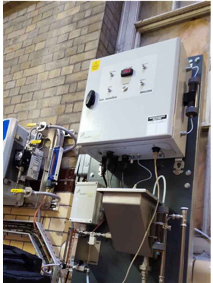
Figure 16. – MS1200 installed in 2014
