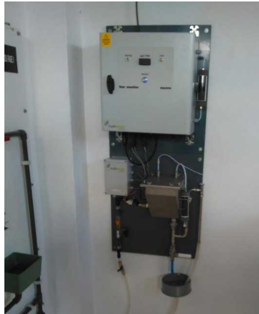
Photo showing the MS2000, the instrument is installed inside the WTP
