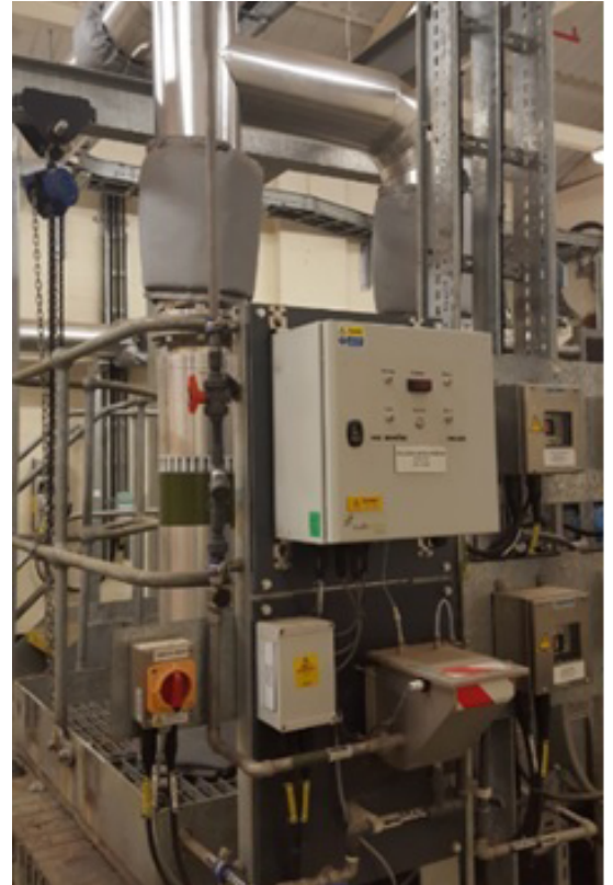
A picture of the unit installed in the factory.
