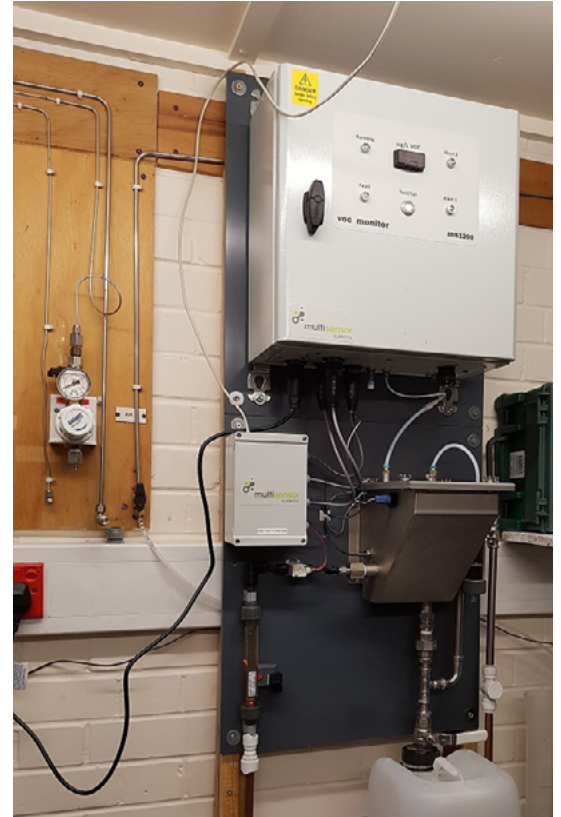
A picture of the unit installed in the outbuilding. The unit is connected to a PLC that records the data and, in case of an accident, triggers an alarm that switches off the intake pumps.
